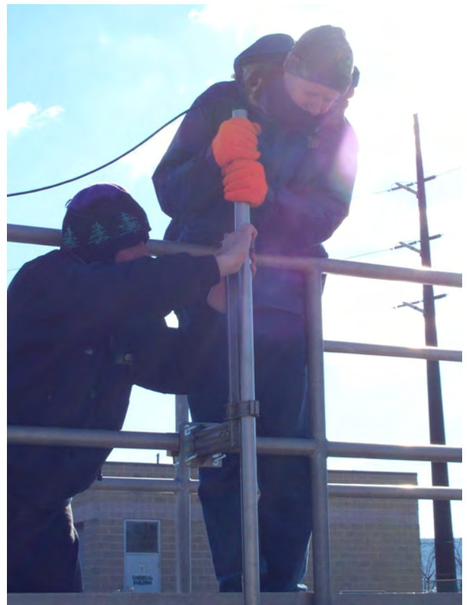
Kevin Anderson, an environmental group manager for the Pennsylvania Department of Environmental Protection, helps to install a sludge level probe at the McConnellsburg Sewage Authority on the coldest day of the year. Marc Austin Neville
